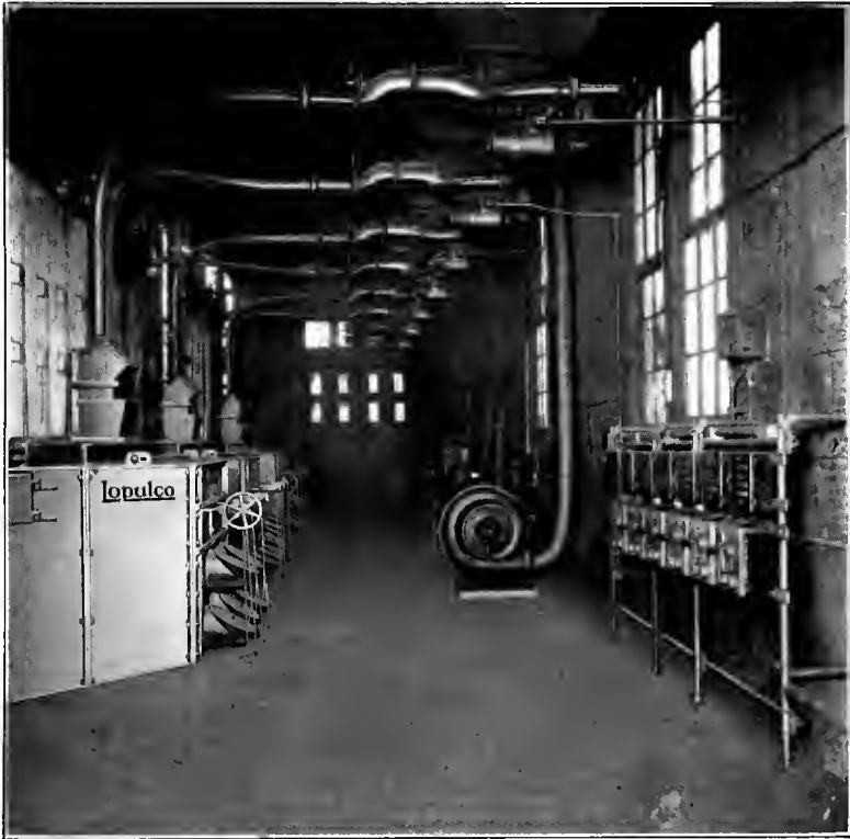
FIG. 112.—Oneida Street Plant of the Milwaukee Electric Railway & Light Co.
